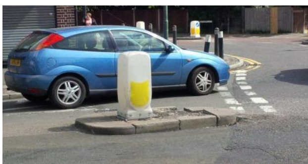
Badly eroded traffic isle. A candidate for spending part of the identified savings?
